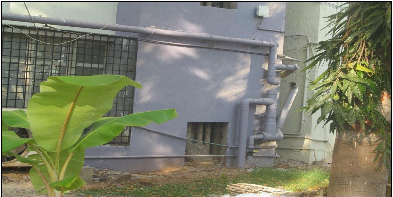
Rain Water Harvesting Pipe line
